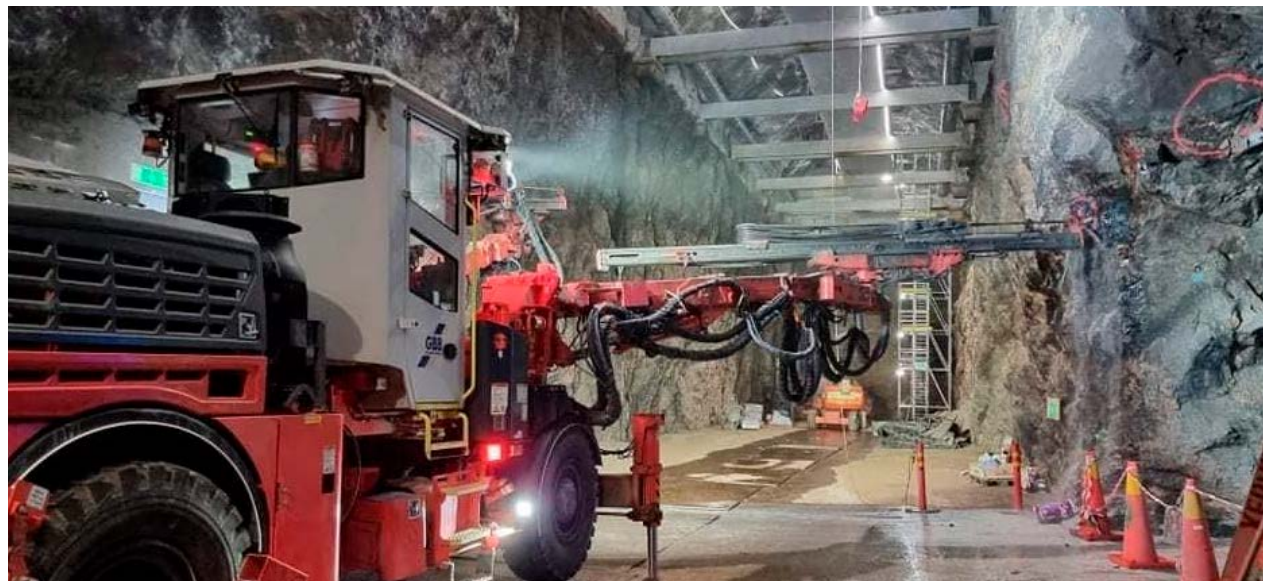
Gnesta Bergbyggare carries out work inside in the Henriksdal water purification plant
